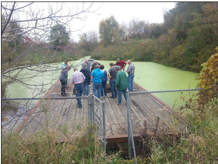
Photos: Outlet Control Structure
